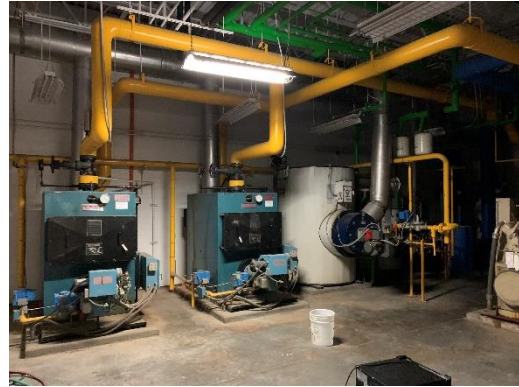
Existing Gas Fired Boilers
