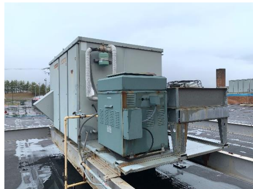
Typical Built-Up DOAS
