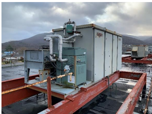
Typical Built-Up DOAS
