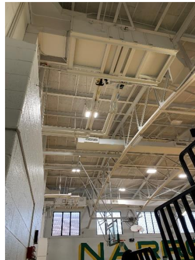
Typical Blower Coil - Gymnasium
