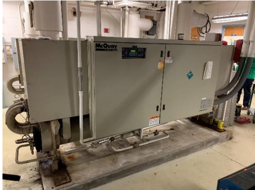
Existing Chiller – 1 of 2
