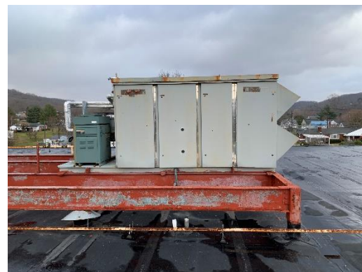
Typical Built-Up DOAS
