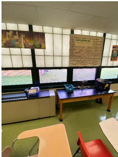
Typical Unit Ventilator - Classroom
