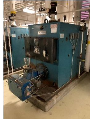
Existing Gas Fired Boiler – 1 of 2
