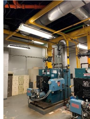
Existing Gas Fired Boilers
