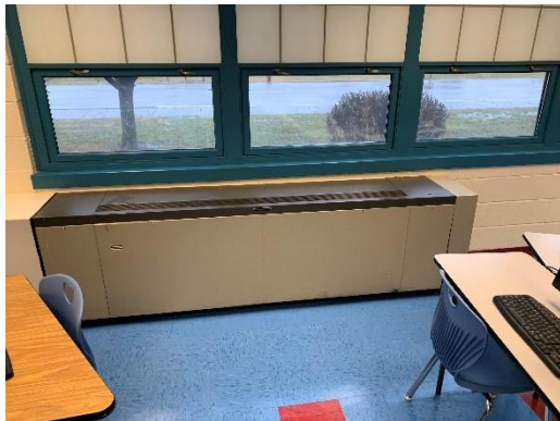
Typical Unit Ventilator - Classroom
