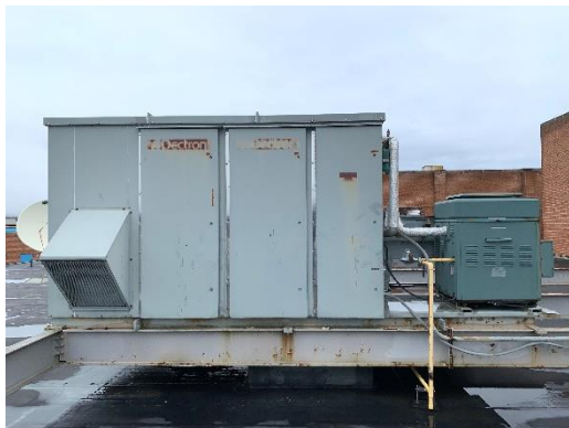
Typical Built-Up DOAS
